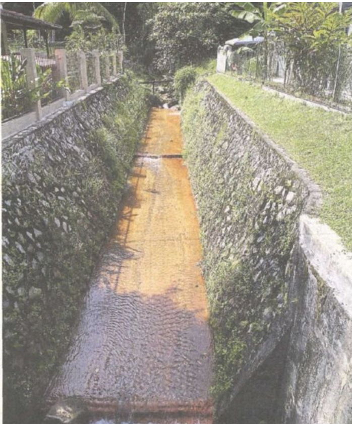
The water from the stream flows into this drain.
